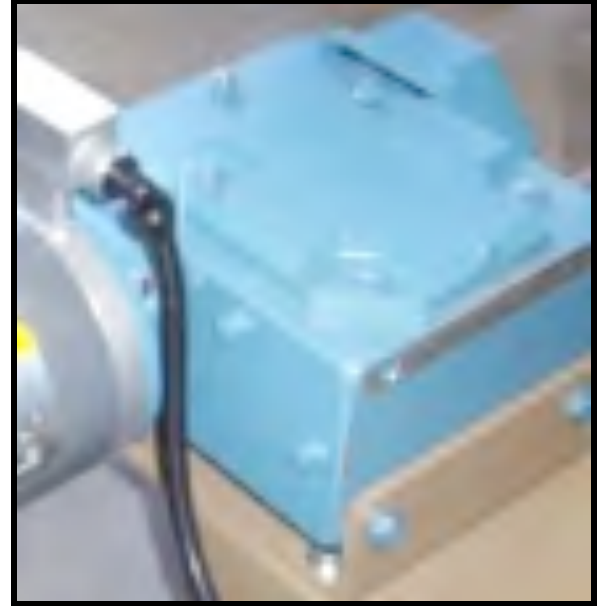
Figure 21 Conveyor Gear Box
