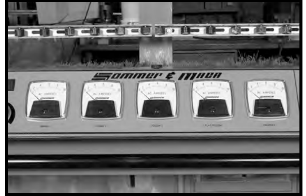
Figure 4 Operator Console Center
