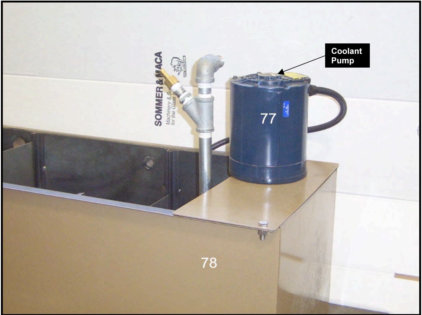
Picture 19 Coolant Tank and Pump
