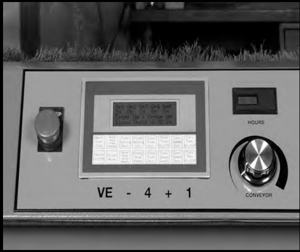
Figure 3 Operator Console Left
