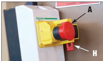
Photo 1. "A" -E-Stop button on main switch. "H" Lockout tab pulls down when E-Stop switch is pushed full in.
