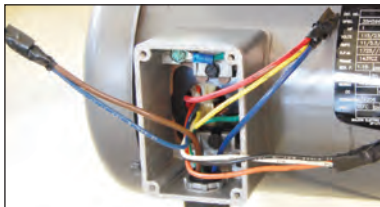
Photo 4. 220 V Motor wiring: •Blue supply wire to Red & Yellow on Motor. •Brown supply wire to Blue on Motor •Green/Yellow Earth wire to earth screw in box. •Black, White, Orange Motor wires together. Secure with screws and nuts and electrical tape.
